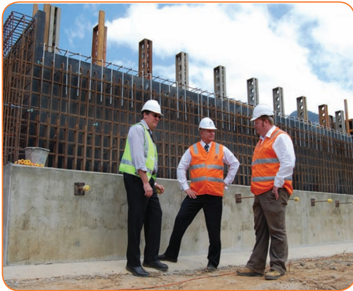
Inspecting the new Mulgrave River bridge progress are Main Roads former Acting Regional Director (Cairns) David Atkinson, Minister for Main Roads Warren Pitt and Main Roads Project Manager Gary Hicks
